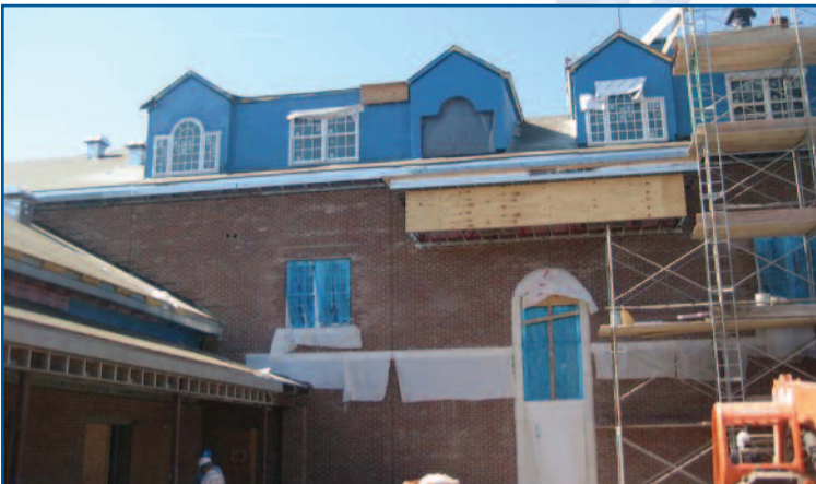
View of the back of the house from the courtyard. Notice the center space reserved for the Edgar Earl Garrison memorial window, which is currently undergoing professional restoration.
