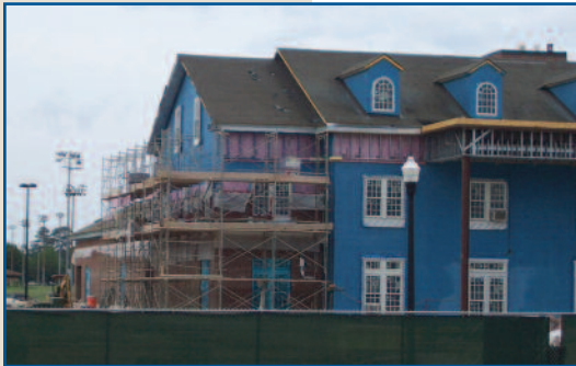
The brick façade is beginning to show on the left side of the chapter house.
